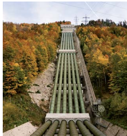
Pressure pipelines of a pumped storage power station
