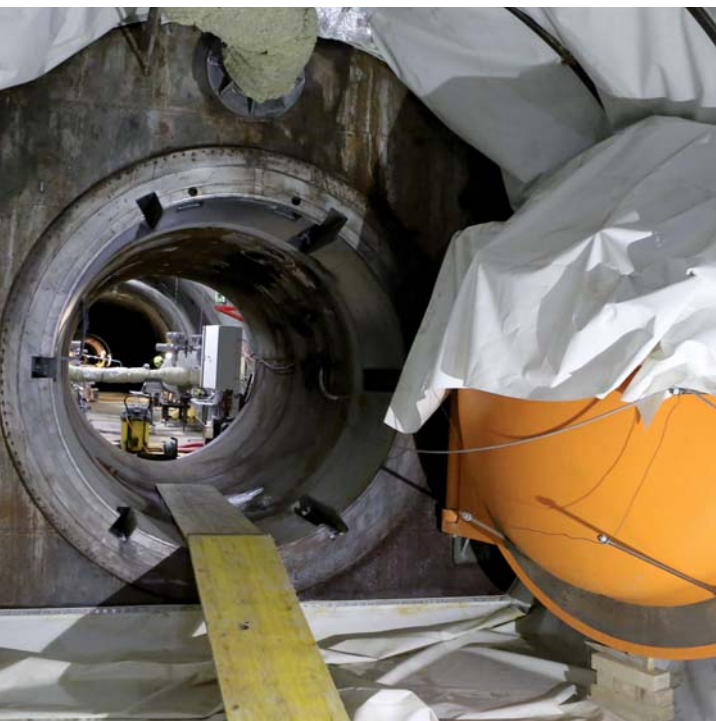
The storage capacity for compressed air is limited by a concrete insert with a diameter of 5 m and by a metal door
