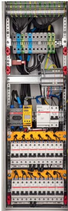
IT distribution board with insulation monitoring device isoMED427P
