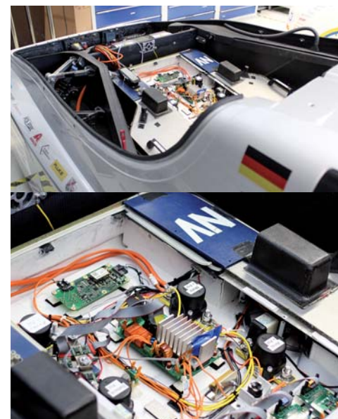
Bender insulation monitor in the battery box of the “thyssenkrupp SunRiser”
