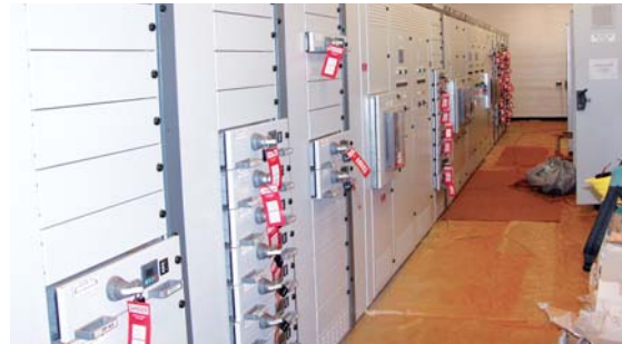
Area 350 switchboard room
