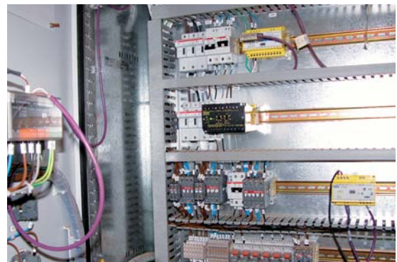
Inside Area 350 switchboard room
