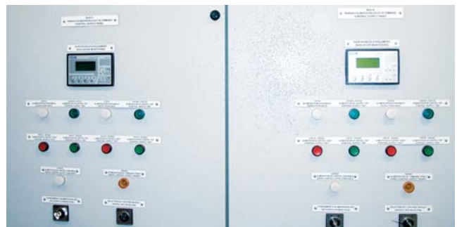
Two of three monitors in operation
