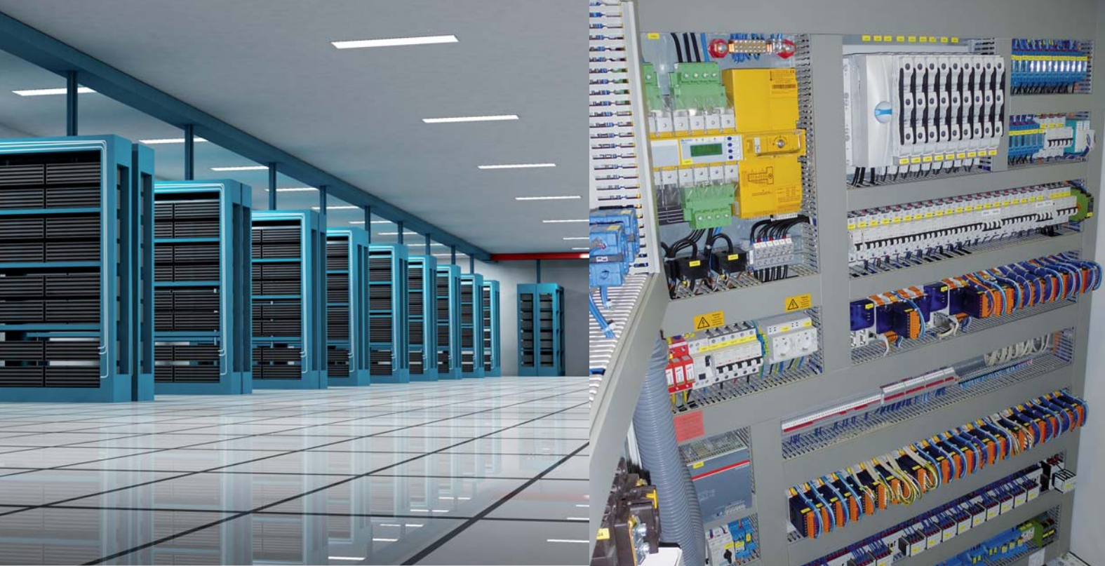
Transfer switching device of the ATICS® series in use
