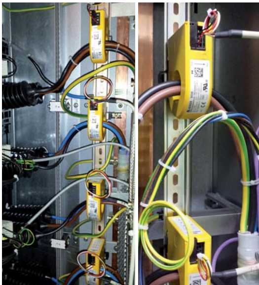
Fig. 2: Cable terminal compartment of a block distribution board with residual current transformers
