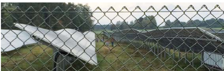
Unauthorised people (family with children) are walking around in the solar field without knowing the dangers lurking around.
