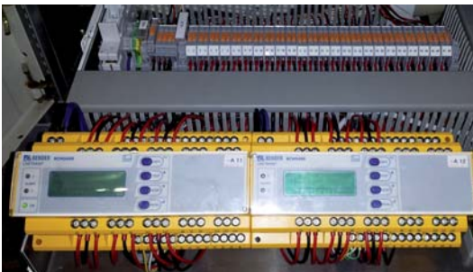
Fig. 3: Overview image of monitoring system of the power plant Waldshut with details of monitored operating material
