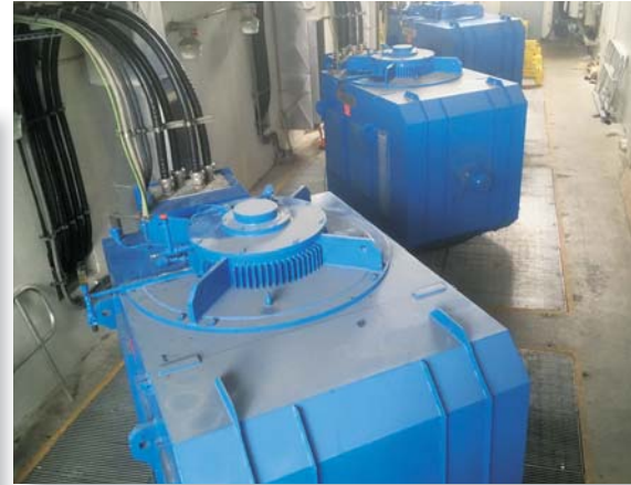
1200 hp influent pump motors
